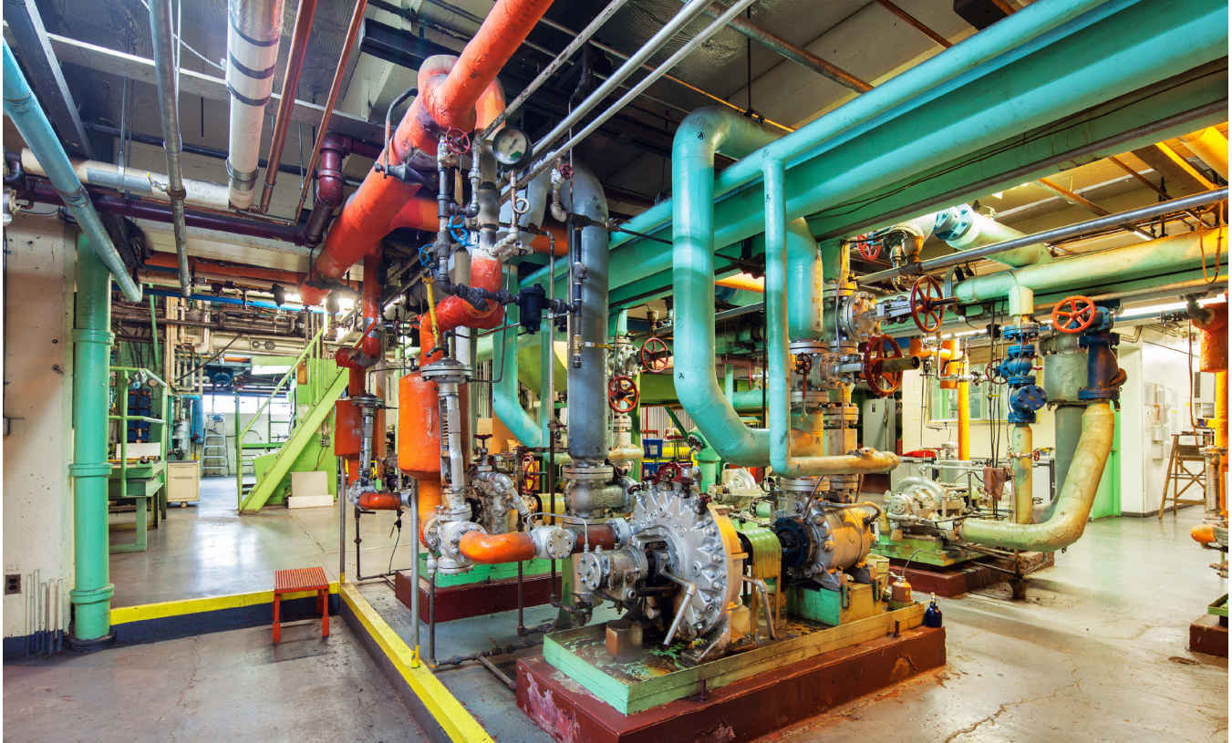
Inside the Creative Energy steam plant at Georgia and Beatty in downtown Vancouver.
